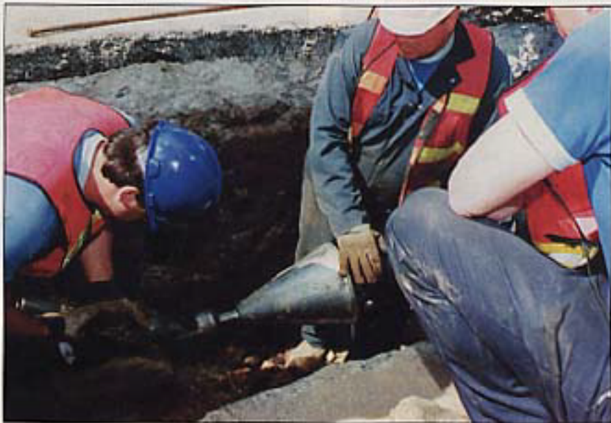
After the Bullet has split the original main, Brooklyn Union employees prepare to insert spreader that clears a path for plastic pipe to follow.
